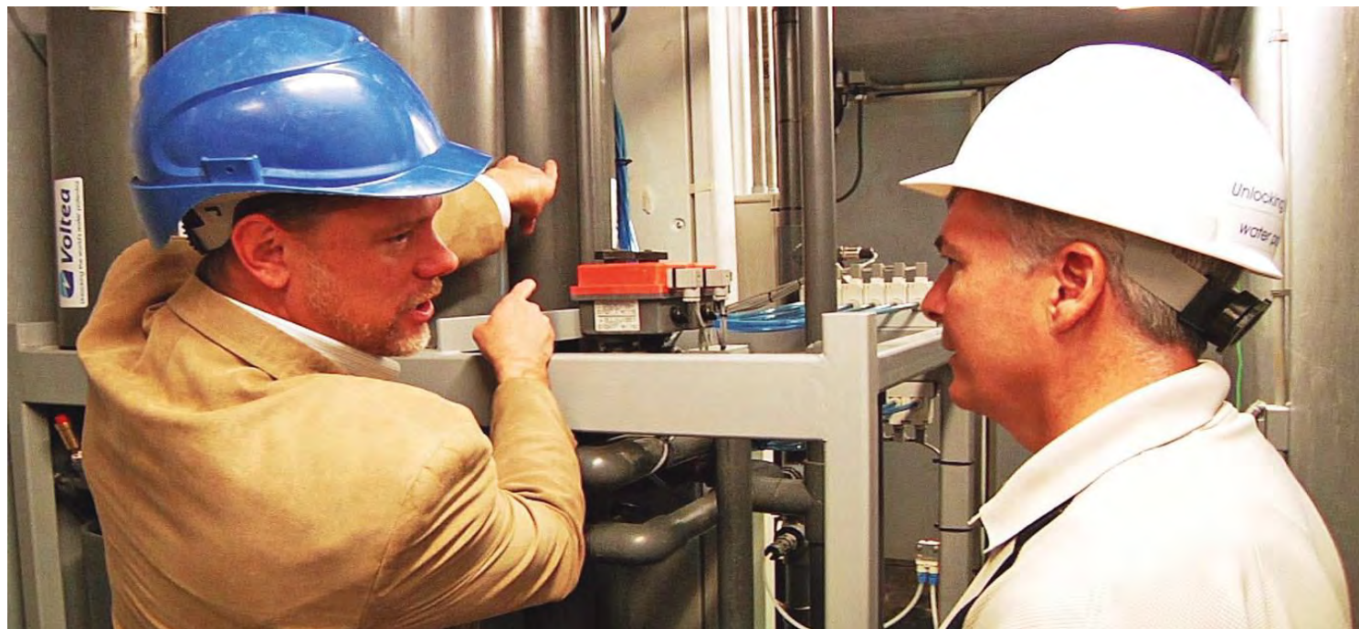
Voltea CEO Bryan Brister and Tim Fitzgerald, a distributor of the electrodeionization technology, work on-site at Republic Steel in Lorain, Ohio.
