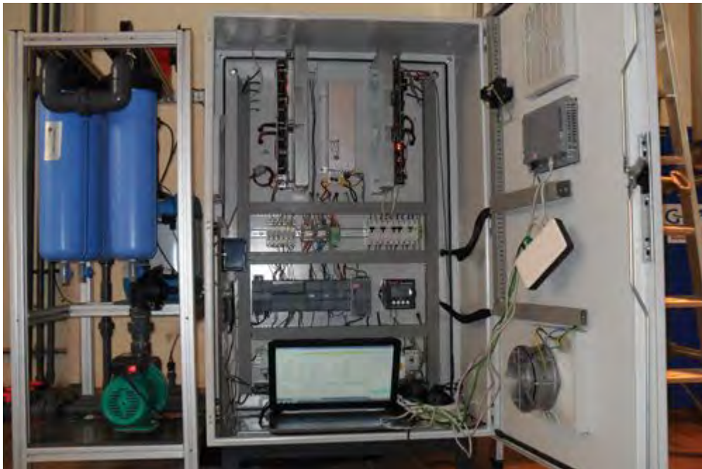
A look into the internal panel box of the CapDI IS2 System, installed at the Unilever plant in Pratau, Germany.
