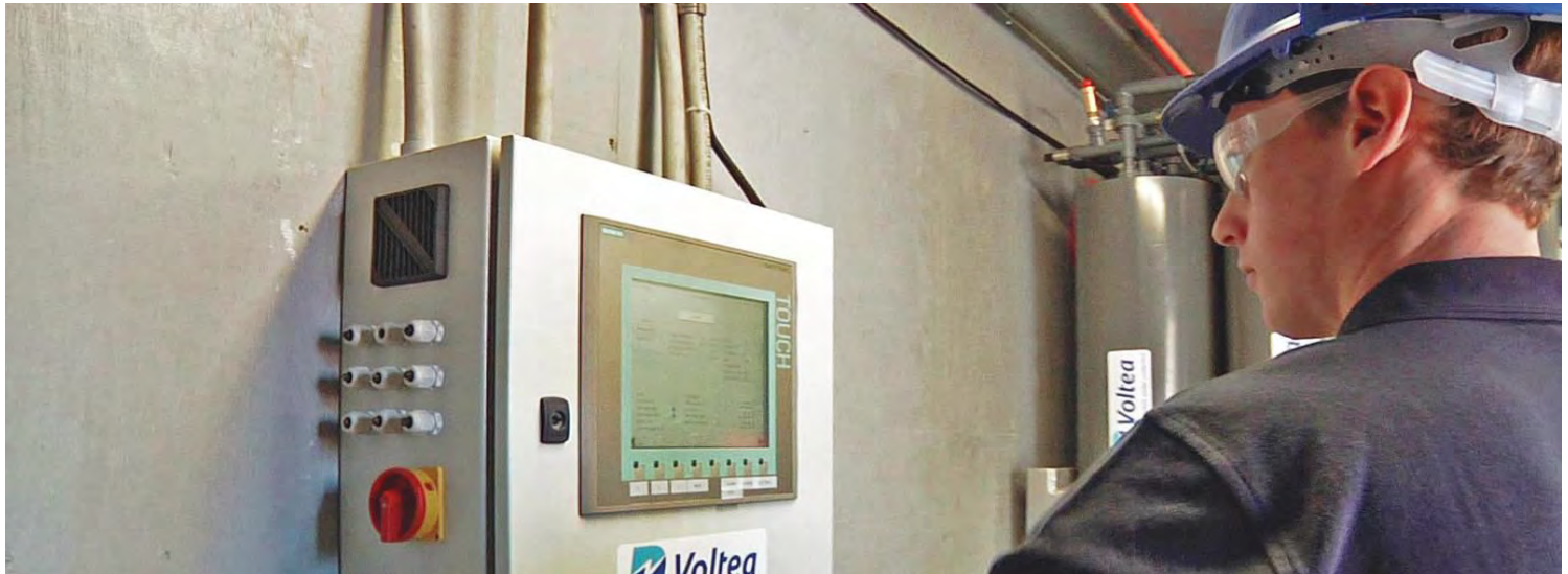
Josh Summers, a field service engineer, manages the control panel of the industrial water treatment system at Republic Steel.
